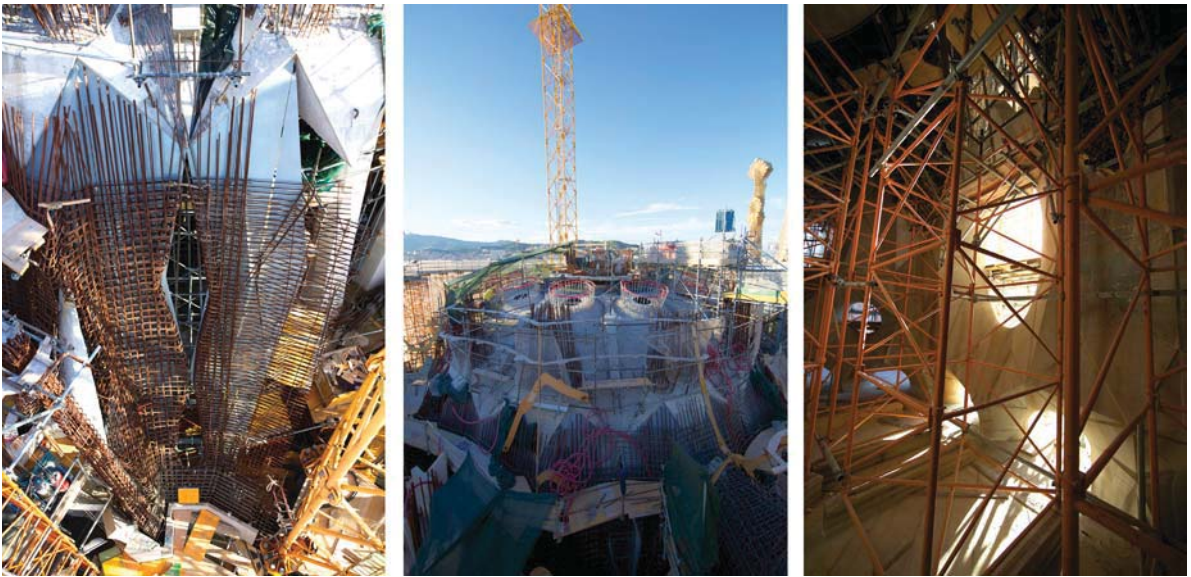
FIGURE 26.16 Looking down at the removable interior formwork. Once the reinforcement is in place, preassembled stonework is lowered in place prior to concrete being poured within (left). Exterior of the Sala Creuer nearing completion (middle). A hint of the intended light effects as the space nears completion (right).
