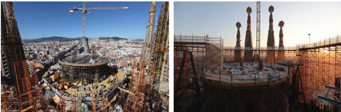
FIGURE 26.10 The formwork for the Sala Creuer auditorium seen from the crane (left); platform used to marshal the precast and cut stone elements (right).
