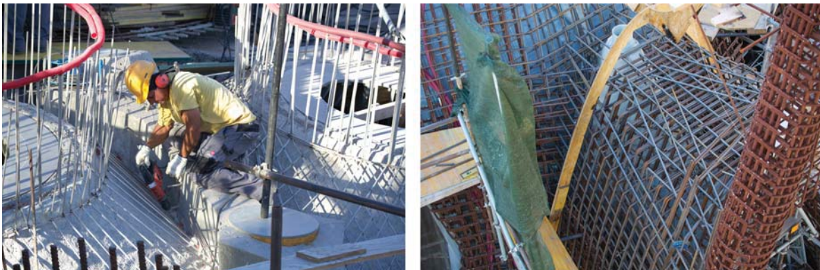
FIGURE 26.15 Exterior view of completing the vaults. Note the reinforcement exactly follows the straight-line rulings of the constituent hyperboloid of revolution geometries (left). Each rebar is drawn in 3D in Rhino (right).
