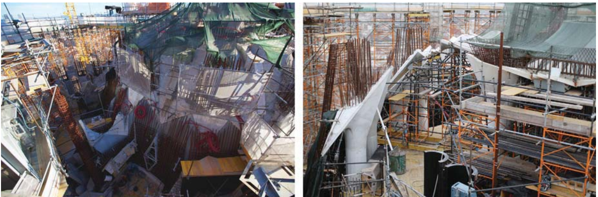
FIGURE 26.13 Looking down toward the nave roof construction (left); column capitals joining the perimeter of the ceiling vaults within (right).
