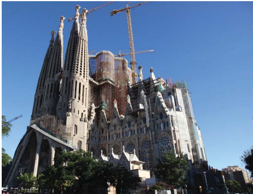
FIGURE 26.17 View from Passion Façade looking up to the Sala Creuer construction from ground level.
