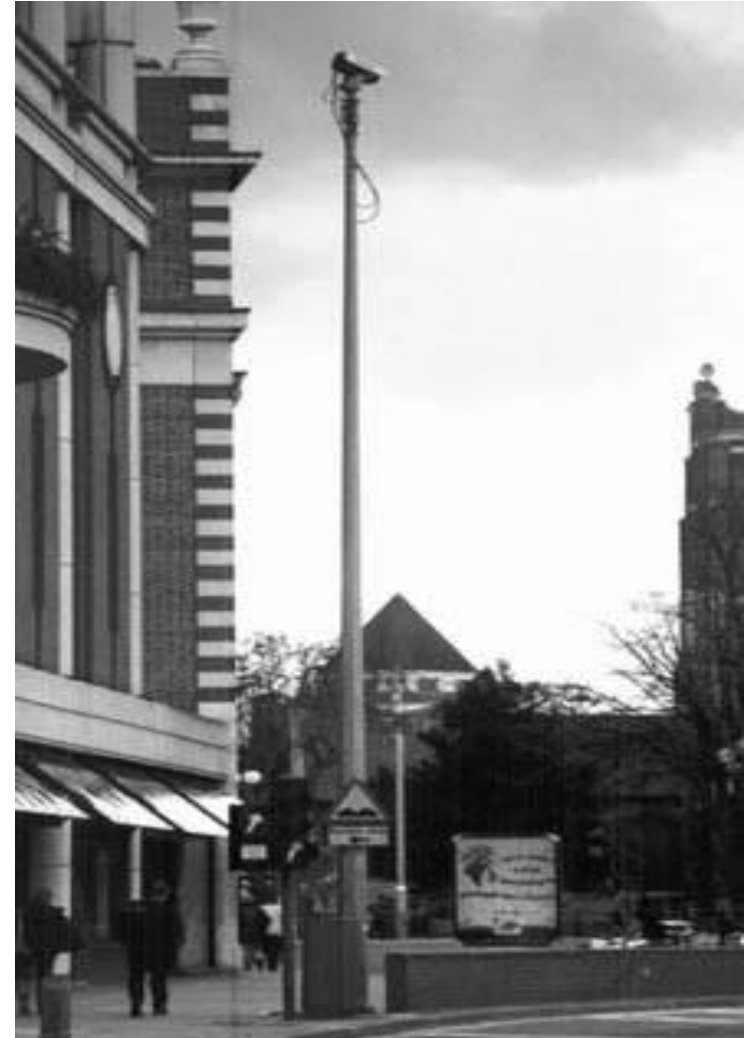
post mounted CCTV
