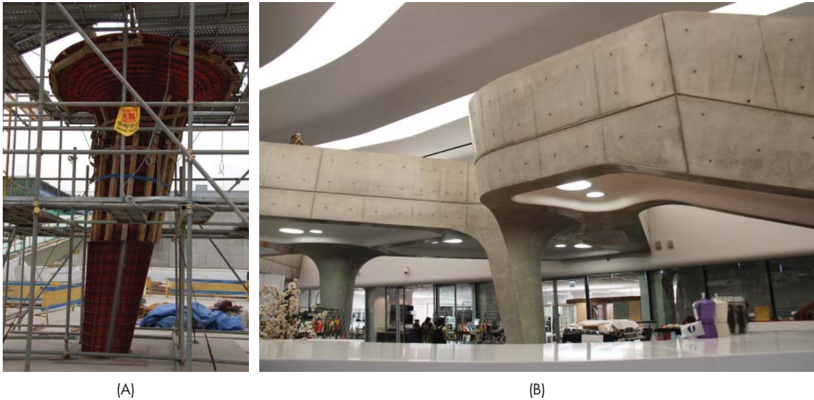
FIGURE 10-4-12 Use of MPSF in concrete work: (A) Assembled concrete forms fabricated using MPSF. (B) Exposed concrete structures.
