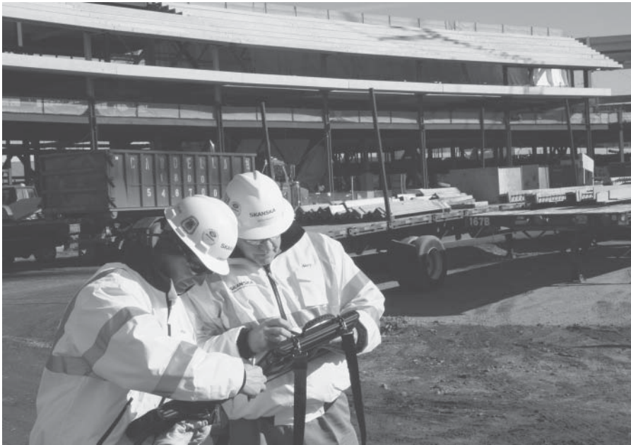
FIGURE 7-9 (Top) Field personnel use rugged tablet PCs to query information about precast pieces and their production, delivery, erection, and approval status from a color-coded model of the stadium. (Bottom) The PCs are equipped with readers to capture information from RFID tags attached to the precast concrete pieces.
