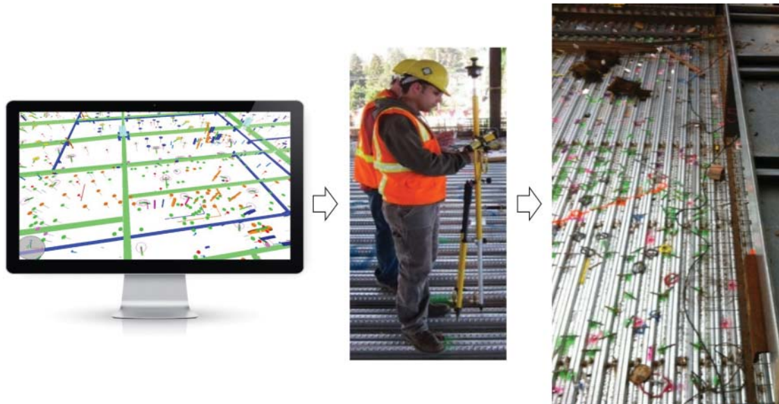
FIGURE 6-18 From model to field: layout of hangers for MEP installation in a flex deck slab shutter system prior to pouring concrete.
