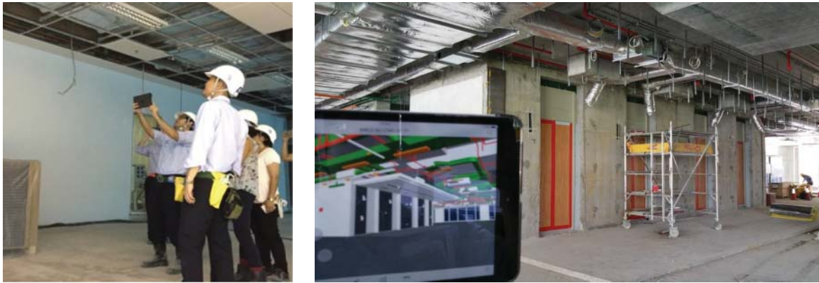
FIGURE 6-15 Viewing HVAC ducts in the BIM model on an iPad on site using the BIM 360 Glue app, during construction of the Mapletree Business Park II, Singapore. See Case Study 10-8 for more information on this project.
