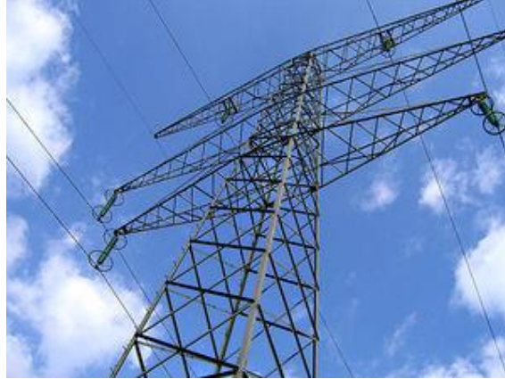
FIGURE 4.3. High voltage power lines are used for the transmission of electricity over long distances.
